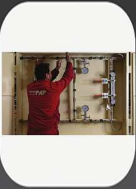
SAMPLE POINT, COOLER, CONNECTION
